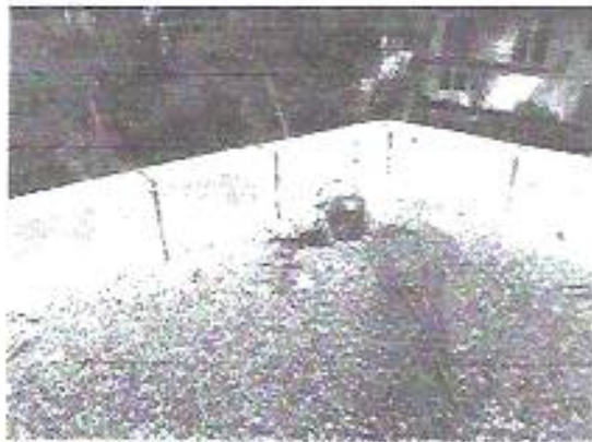
Injection gaz traceur
