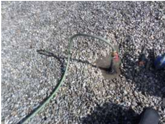
Injection gaz traceur
